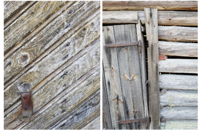
Figure 7 Examples of uncoated timber structures that have been exposed to the effects of weathering for near a century.
